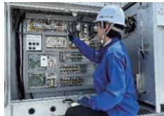
Air conditioner control panel inspection
